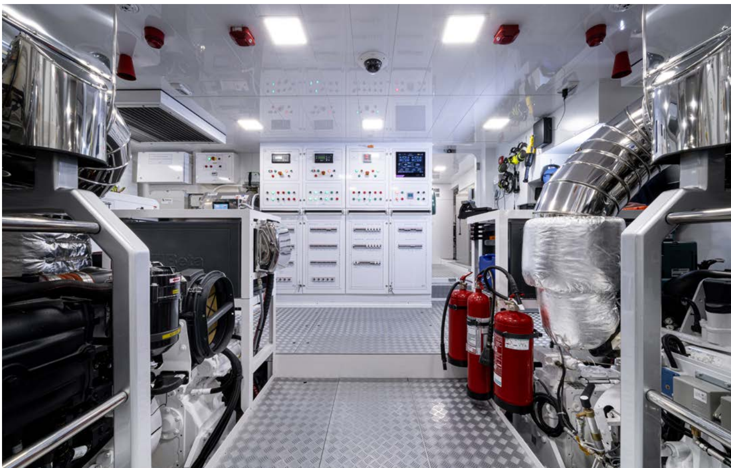
ENGINE ROOM / LOWER DECK
